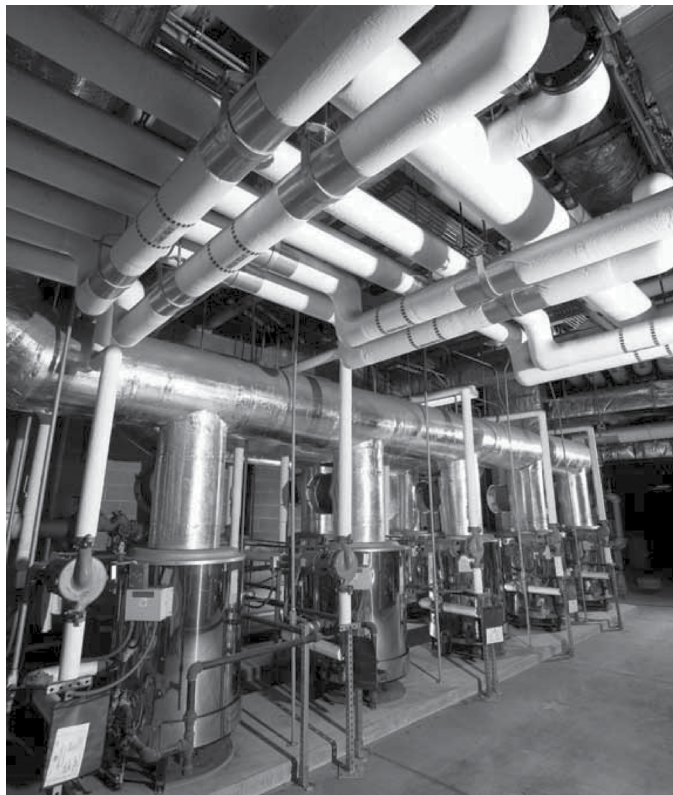
Above: Installation at Cleveland Brown Stadium
